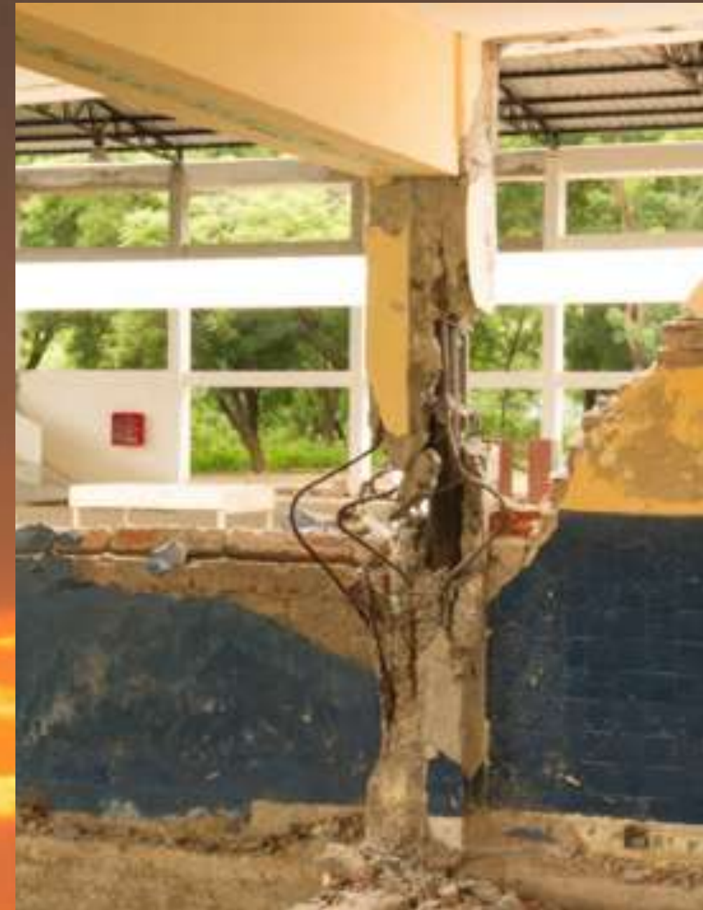
Column failure in school 100k from Epicenter of Quake
