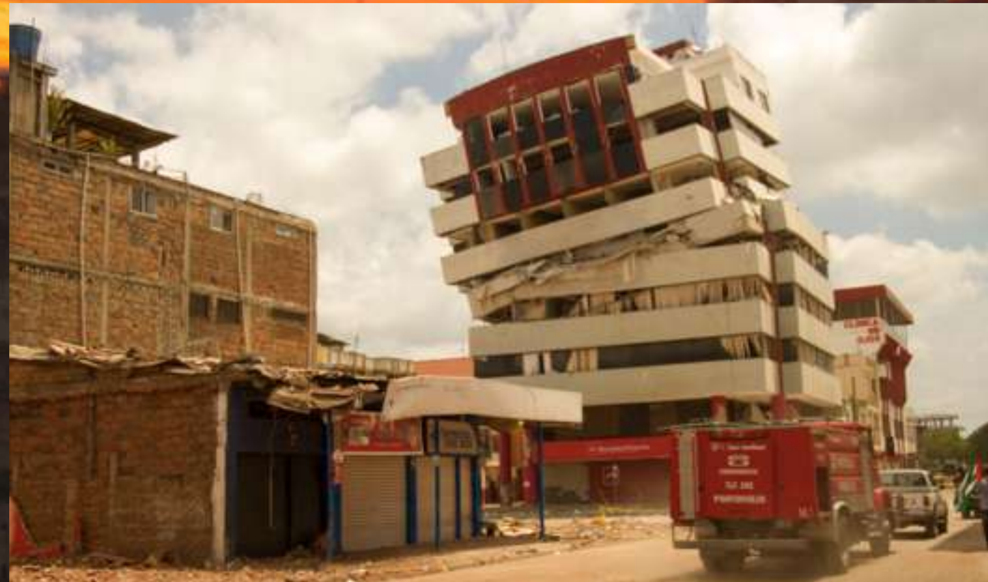
Mid section Structural Failure on office building 100k from Epicenter of Quake
