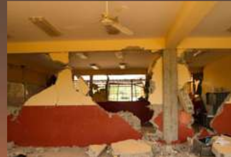
Non Structural wall failure 100k from Epicenter of Quake
